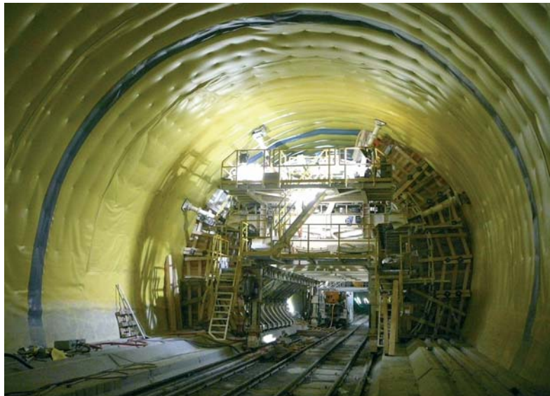
Fig. 4 Gewölbeschlagen. Montage der Stirnschalung (© Arge Transco). Lining formwork car. Installation of the bulkhead formwork (© consortium Transco).
